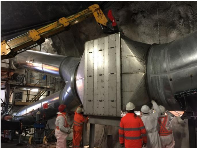
Droplets removal system for an aspiration duct inside a tunnel
